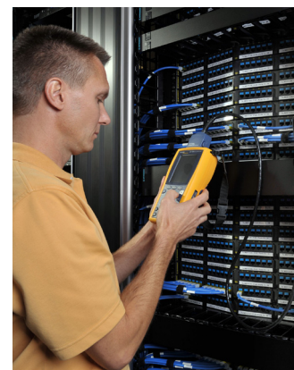
Terrance Electric used Fluke Networks’ DTX CableAnalyzer to certify the new installation to 10GBASE-T. Multiple two-man teams were used to test and document over 40,000 links.
