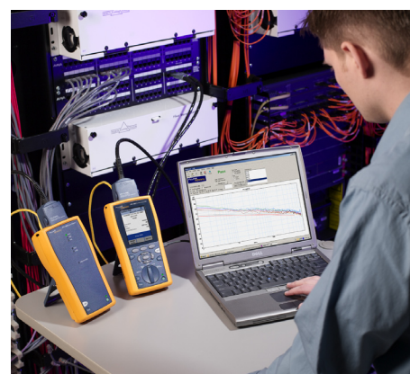
The DTX CableAnalyzer test multiple “victim” links for alien crosstalk during 10 Gigabit/s Ethernet testing. Results are quickly analyzed and stored on a laptop, providing complete documentation of this phase of the 10 GB/s test process.
