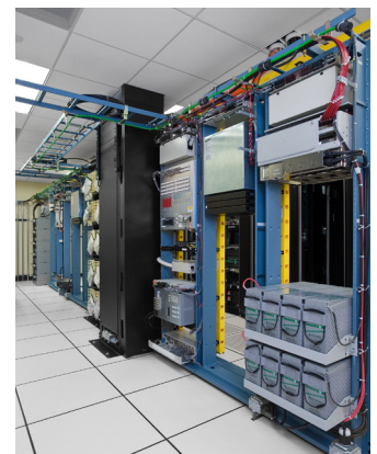
The cable installation at HSBC headquarters was designed to be both state-of-the-art and future-proof. High performance and energy efficiency were key element of the data center design.
